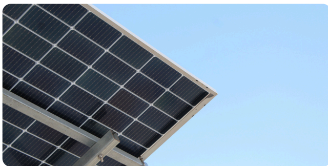
Solar Panels at School
